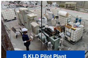
5 KLD Pilot Plant
