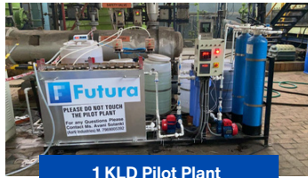
1 KLD Pilot Plant
